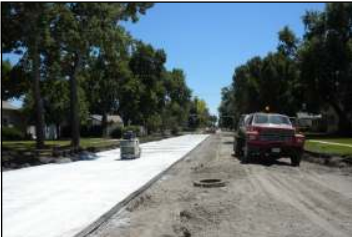
Paving: Black, Joe, and Don's crew working on the 5 th Avenue project in Kearney.
